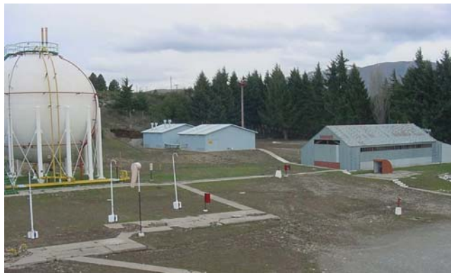
Photo 1: SNG Peak Shaving System, Bariloche, Argentina (Photo courtesy of Camuzzigas, Argentina)
