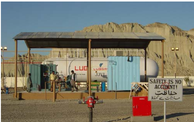
Photo 3: SNG Blending system installed at Gwadar, Pakistan (Photo courtesy of SSGC, Pakistan)
